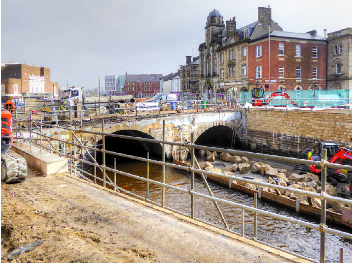
FIG. 1 Ongoing work to the Rochdale Bridge during the Revealing the Roch Project: February 2016. Source: ©David Dixon https://www.geography.org.uk/profile/43729 and licensed for reuse under CC-BY-SA 2.0 via geography.org.uk
