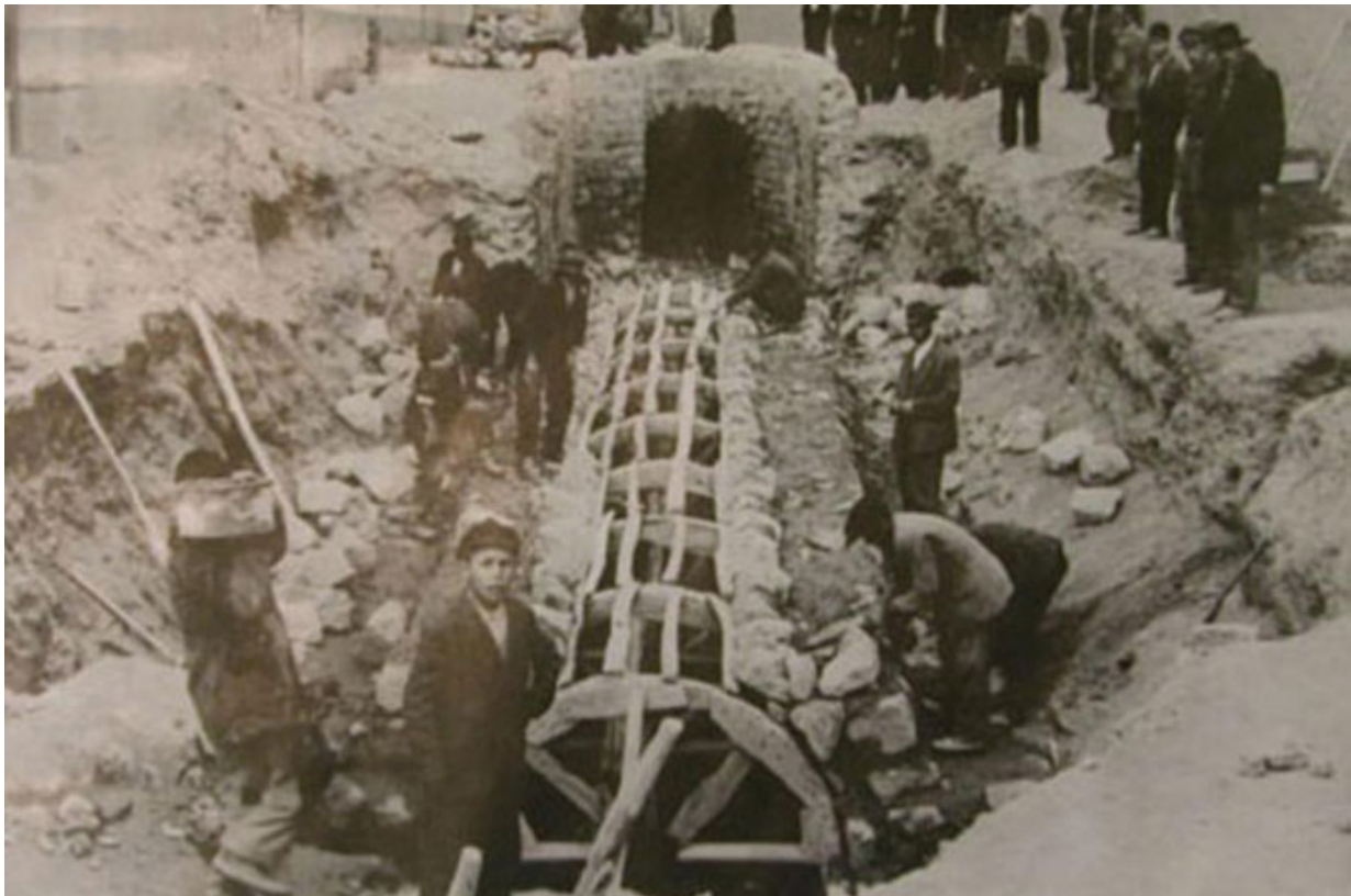
FIG. 5 Preservation and maintenance of one of Tehran's qanats during 1915-1918 period by local citizens. National Library and archive of I.R.I
