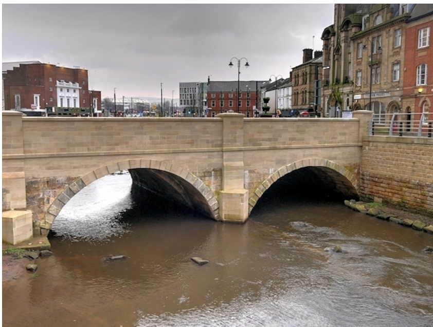
FIG. 6 Rochdale Bridge following restoration, 2017. Source: Copyright David Dixon and licensed for reuse under CC BY-SA 2.0 via geography.org.uk.
